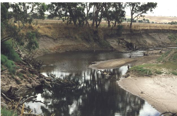
Photo 75 (above) – ‘improved’ Wannon, 2 miles below Sandford Bridge - eroded banks (Feb. 1977)
